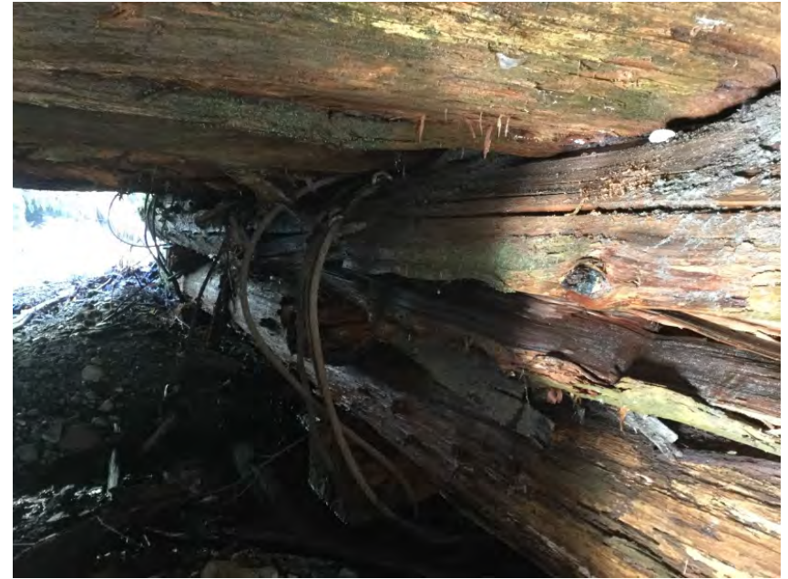
Top face log on left abutment crushing
